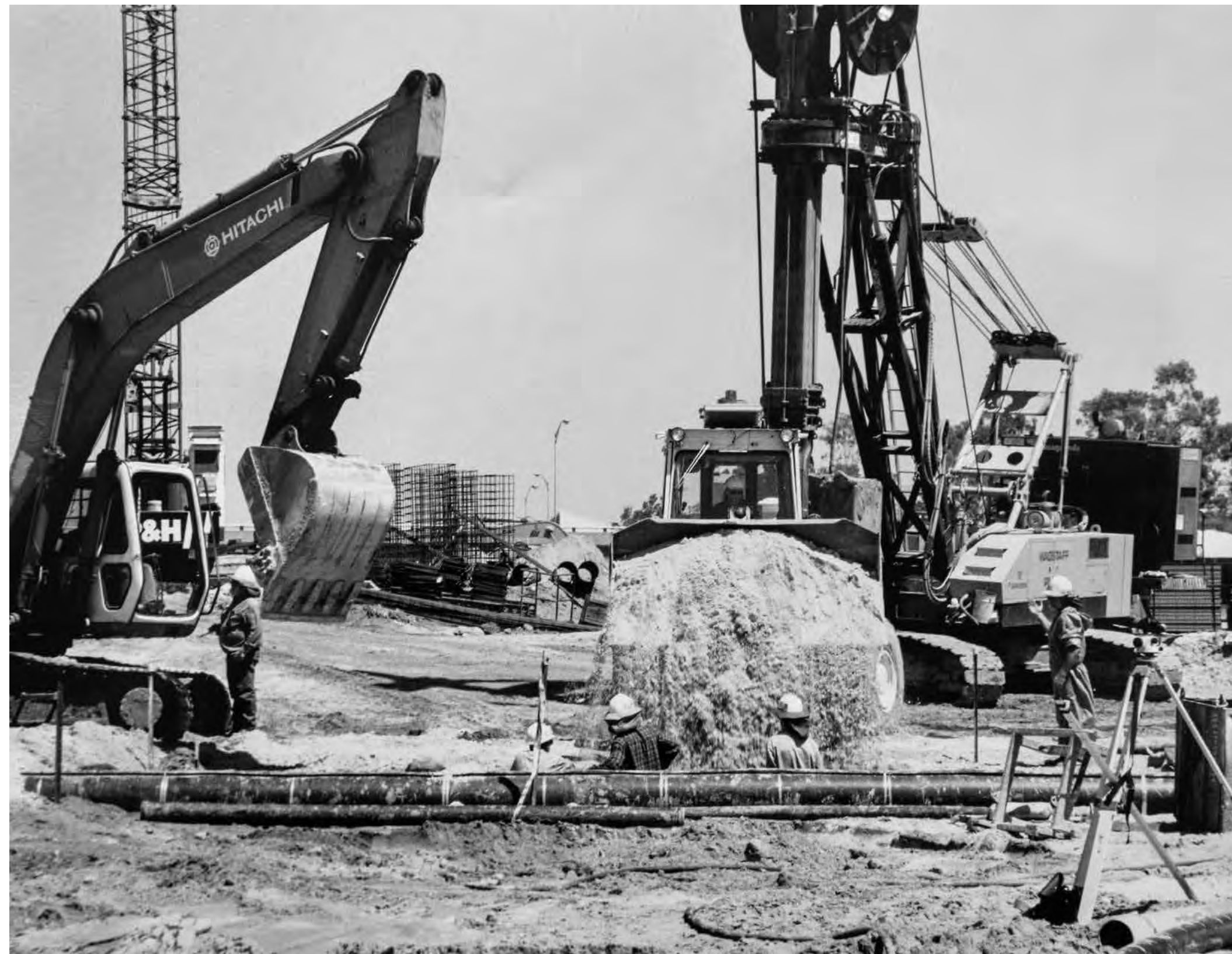
Images (left and right) courtesy of Main Roads WA - Graham Farmer Freeway construction
